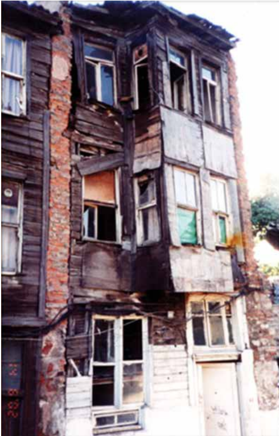
Figure 11. A ruined house in Zeyrek
