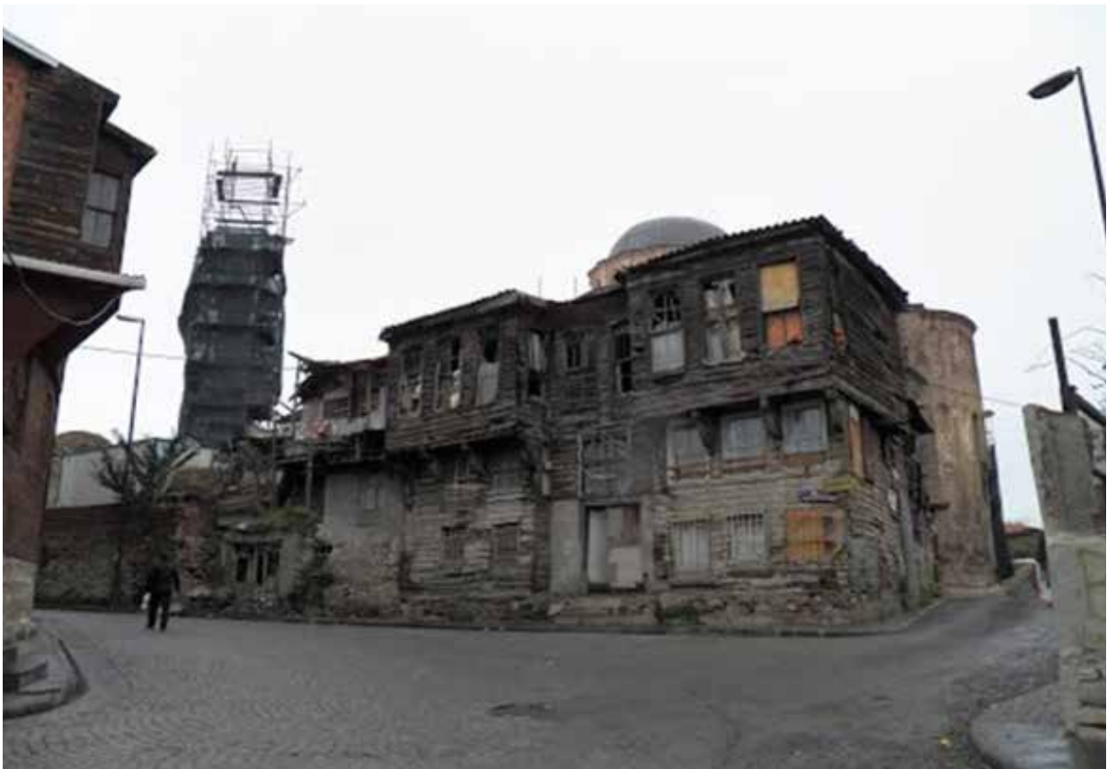
Figure 10. Decay in Zeyrek
